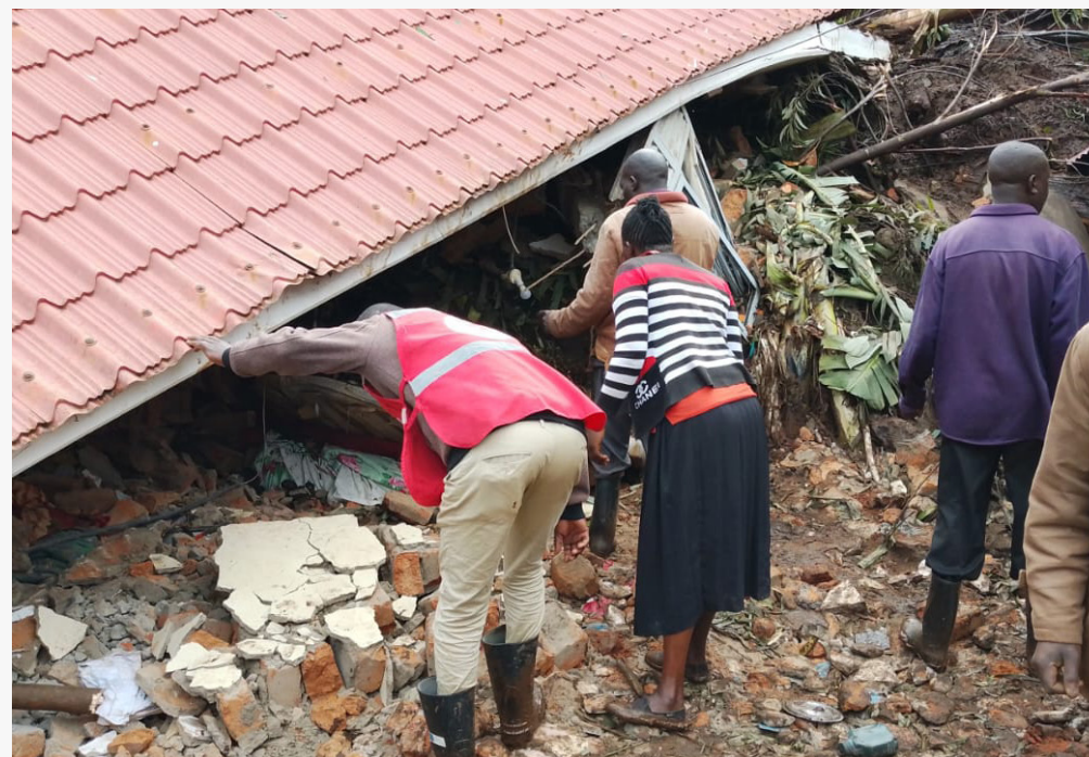
Landslide in Kapsomo Village, West Division, Kapchorwa District, in Eastern Uganda on November 1, 2025. Photo | Uganda Red Cross Society
