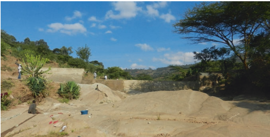
Fig. 6 A newly constructed sand dam by the Kitito Self Help Group, Machakos County, completed in June 2013. The dam has a 17.5 meter spillway. The 1.4 meter high left wing adds an additional 7.7 meters and the right wing another 6.0 meters. It stands 2.8 meters above bedrock and is 1.8 meters thick at the base, 1.0 meter at the top of the spillway, and 0.68 meters at the top of each wing. The entire structure has a volume of approximately 85 cubic meters. The dam was built by hand with more than 100 community members involved in the process. (Photo by author 2013)
